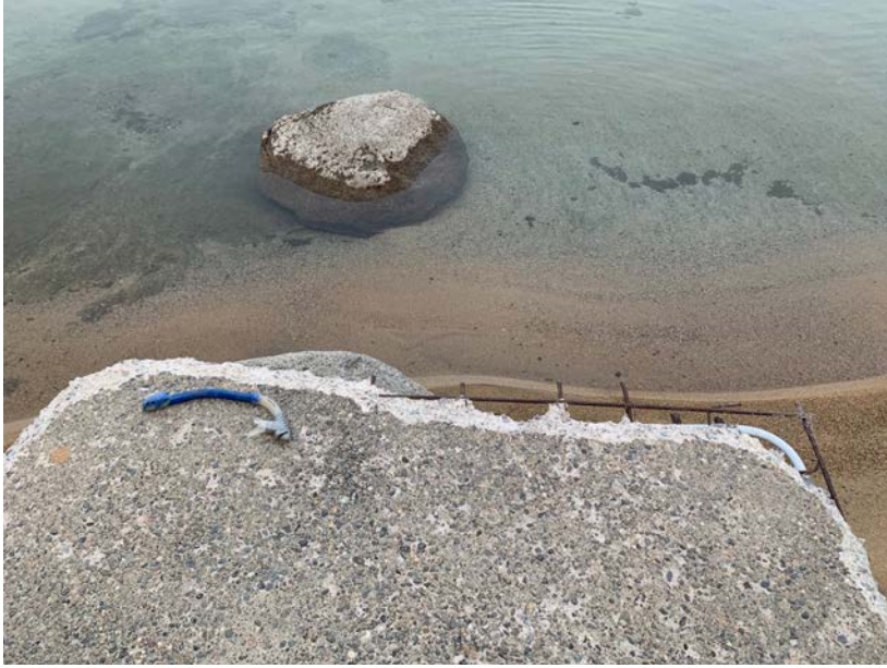
Erosion of Concrete deck and exposed rebar.
